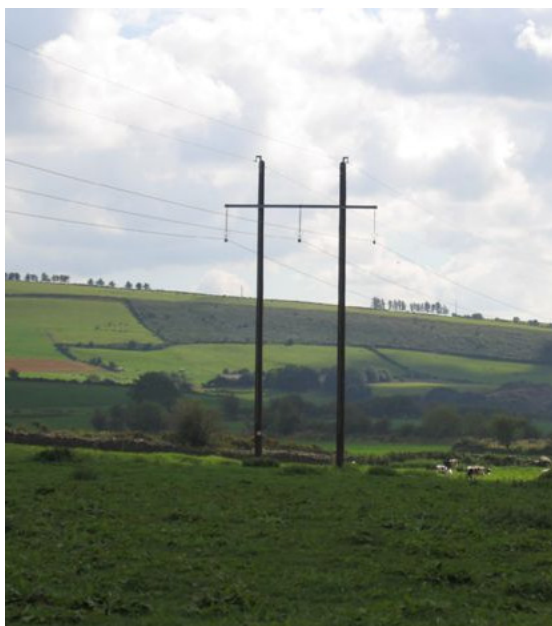
Figure 5: Typical Wood poleset
